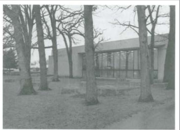
Figure 2. A photo taken prior to construction of the bank addition. The bales of straw are placed where support pillars will be located.
