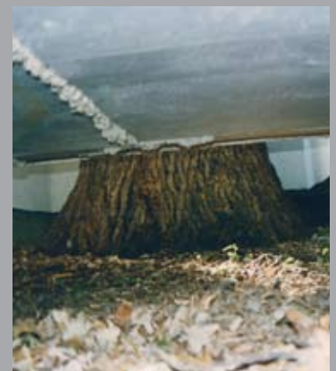
The void beneath the building with its floor supported above the undisturbed soil surface.
