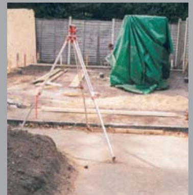
A similar view from the entrance off the public road with the void-former stacked beneath the green sheet ready for use as a temporary floor base.
