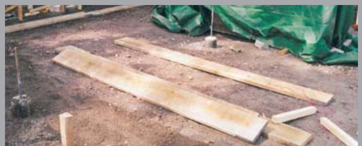
Wooden pegs and boards are the shuttering used to form the temporary side framework for the concrete floor, which will be eventually supported by the piles that can be seen sticking out of the ground.
