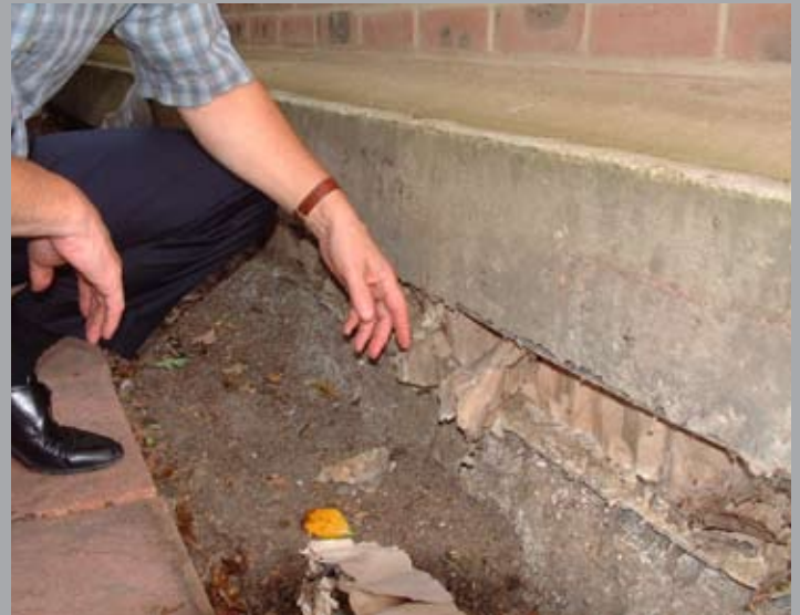
Close up of the floor slab showing the biodegradable void-former layer, resting on the soil surface, which supported the poured concrete of the floor until it had set.
