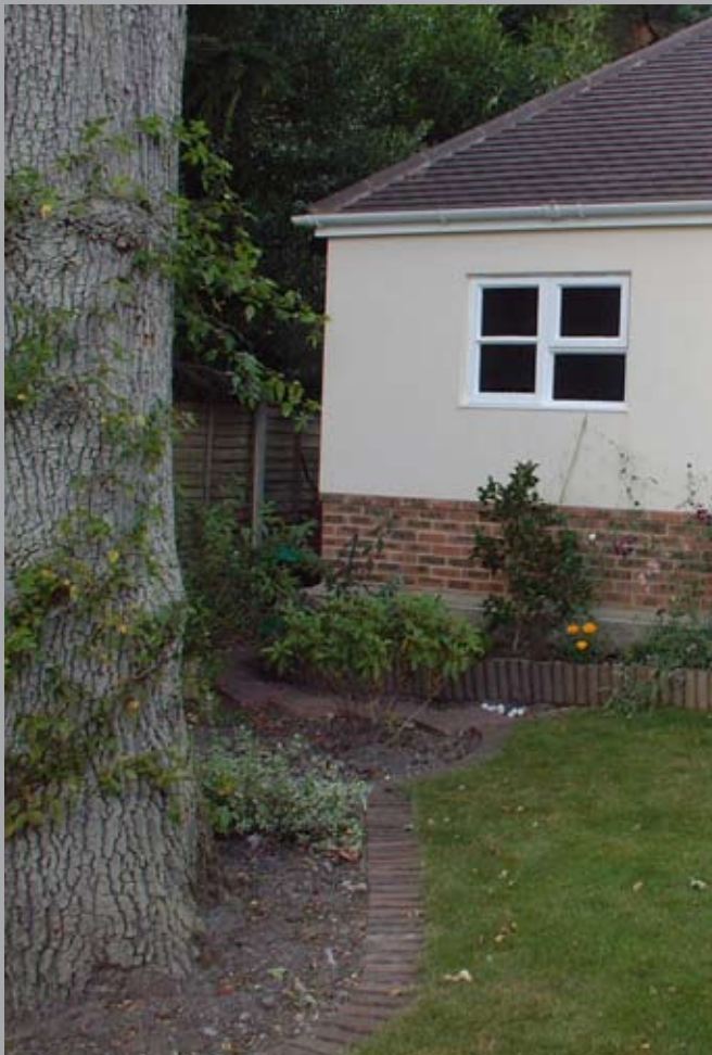
The oak in the foreground with the completed double garage about 4m away.
