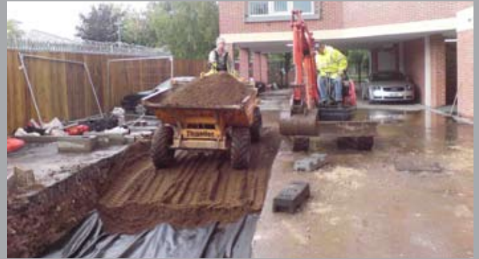
Existing services were covered with a geo-textile membrane and the special structural tree soil filled the planting pit.
