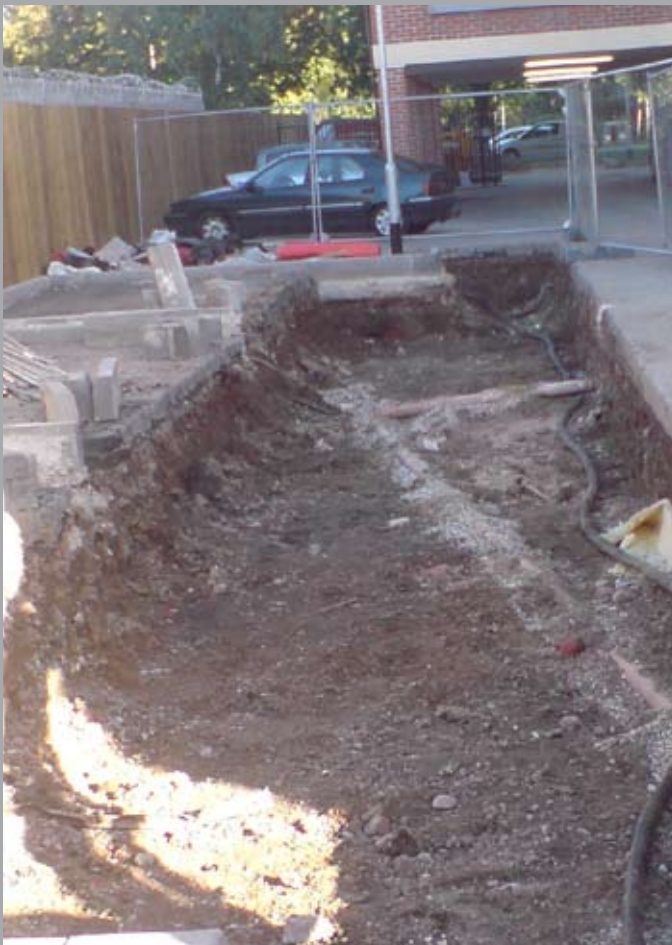
Once the main construction was completed, the linear planting pit was excavated to a depth of 1m in the parking area.
