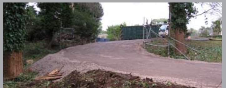
The permeable wearing surface is installed on top of the filled cells and profiled for safe vehicular use.
