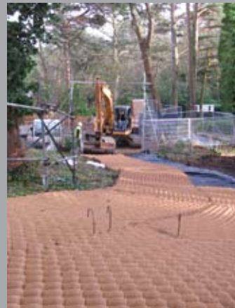
The flexible cells are pinned out onto the soil surface without any excavation.
