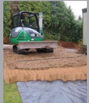
The stone is spread over the area of cells until they are all full, forming an interlocking and rigid grid that spreads the load.
