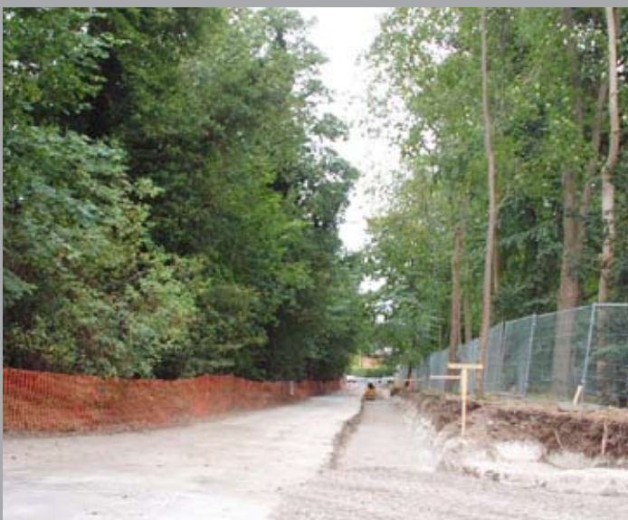
Conventional installation of new surfacing by digging out about 50cm of soil and then filling with compacted stone is not tree-friendly and often results in their removal.
