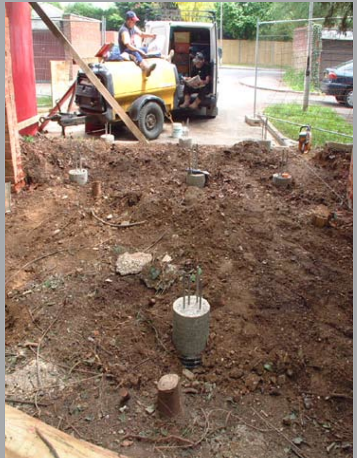
The small diameter piles were installed by a lightweight machine, with their tops sticking out of the ground ready for the fitting of the concrete roadway.
