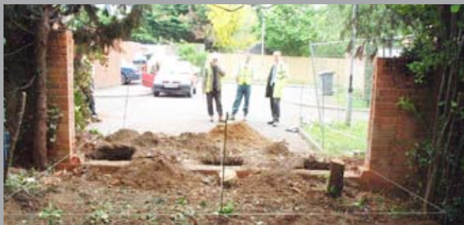
Work started in 2003 by cutting the wall at each side of the access and carefully removing the top, leaving the footings still in the ground to avoid damaging roots. The pile holes were dug by hand to 0.75m depth to ensure that no significant roots had to be cut.
