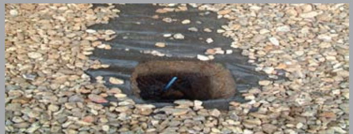
The pile locations were all hand dug to a depth of 0.75m to ensure that no large roots would be damaged. If roots were found, the pile locations were shifted to avoid them.
