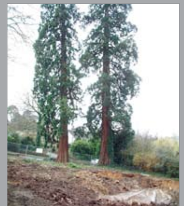
The bungalow had to be carefully demolished ready for fencing the trees to prevent accidental damage to their trunks.
